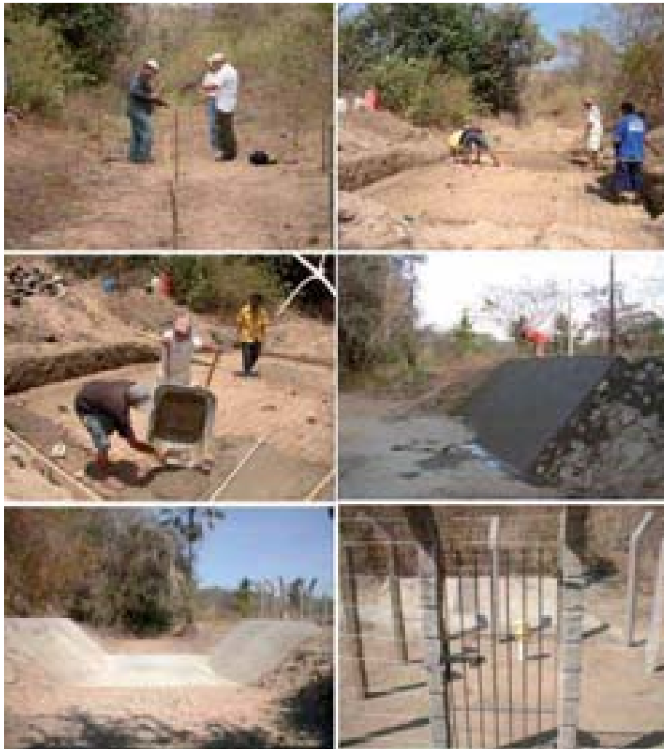
Photo 2.03 – Construction stages of flume 01: plotting, iron structure, concrete application, finish and completion.
