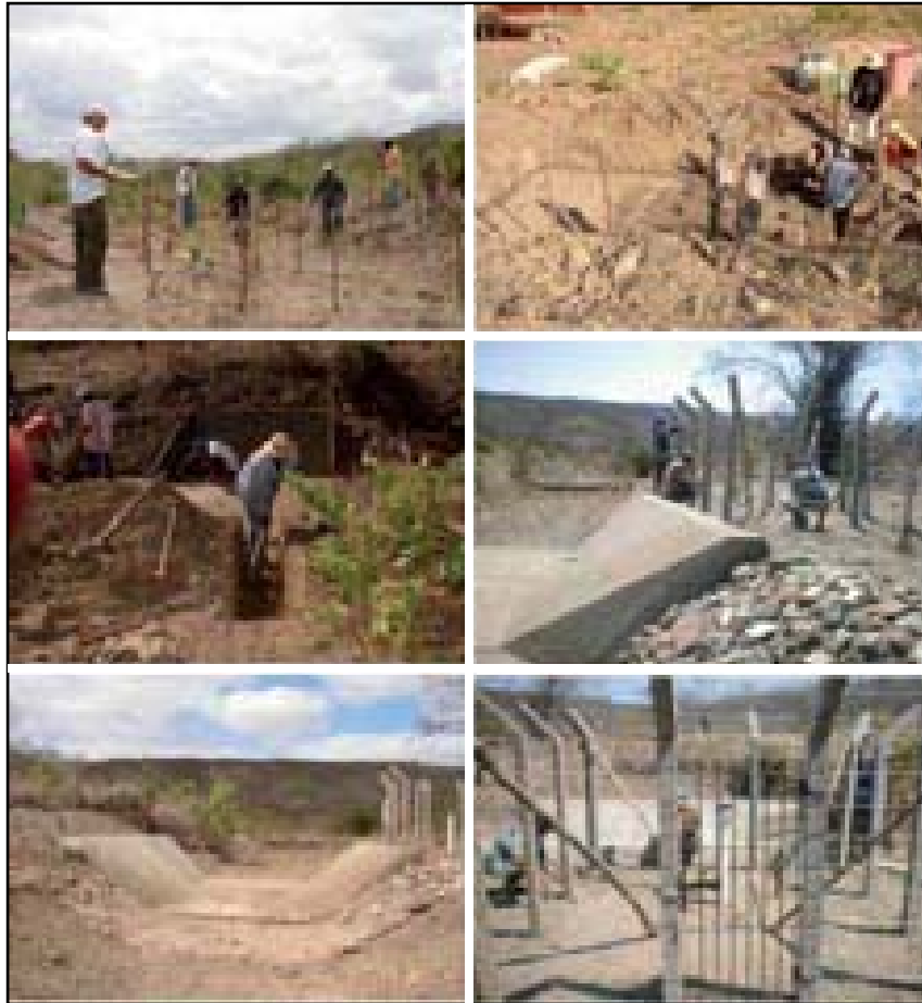
Photo 2.04 – Construction stages of flume 02: plotting, iron structure, concrete application,, finish and completion.
