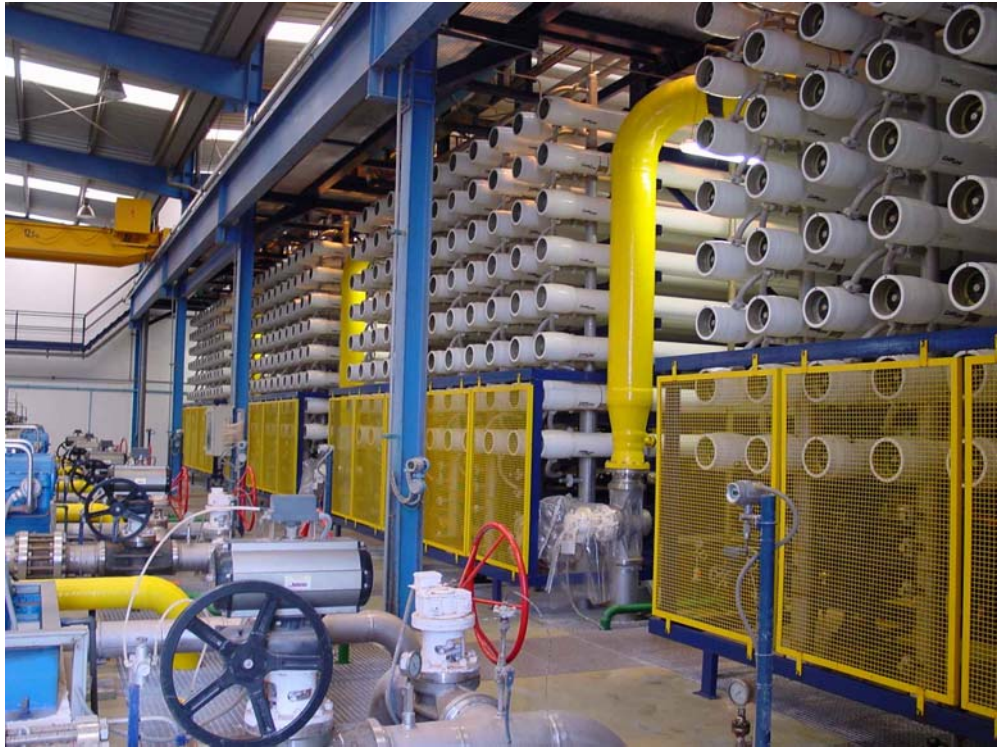
Insular de Aguas de Lanzarote S.A (Inalsa) uses FILMTEC elements to convert seawater to potable water. iLEC interlocking endcaps make the process easier and less expensive. (Photo courtesy of Inalsa)
