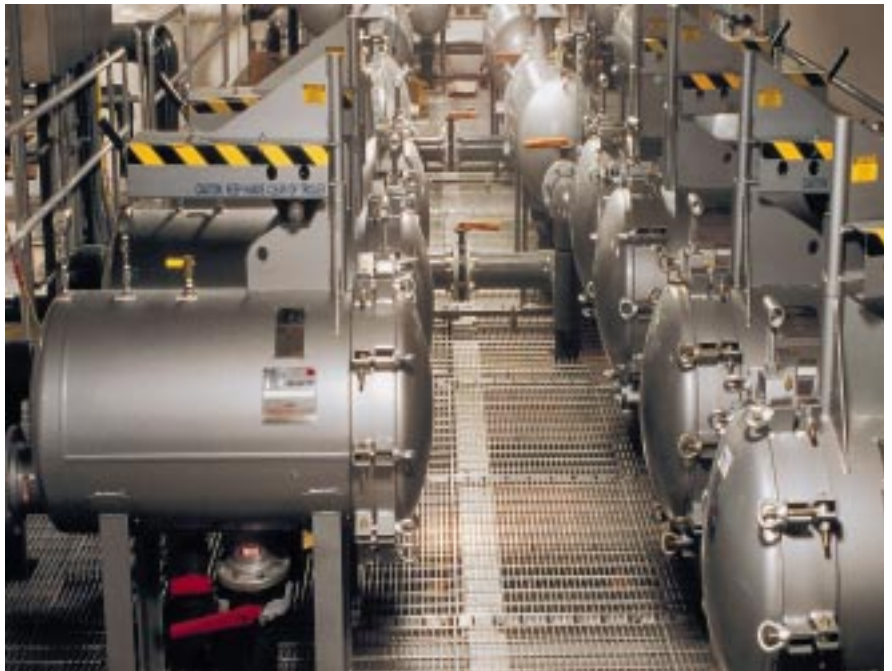
High flow reverse osmosis prefiltration is accomplished with 3M filters in this semiconductor manufacturing plant.
